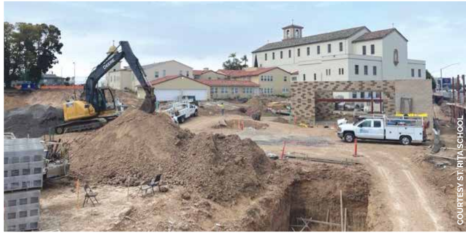
WORK IN PROGRESS: The $7-million "Art, Play, Pray" project is currently under construction at St. Rita School and Parish, where it is expected to be completed this summer.
